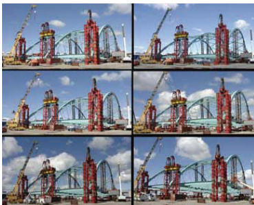
A 400 foot long and 80 foot high section of the new Providence River Bridge moving across a pier at Quonset. Photo courtesy of the CME website www.cmeengineering.com
